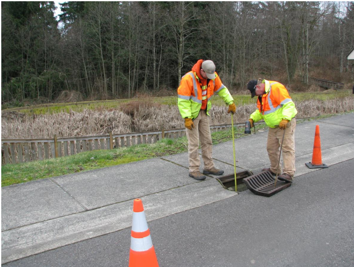
City workers inspect a catch basin that discharges into a storm pond
